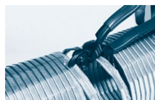
Step 3: Cutting of the protruding profile with a shear blade or diagonal cutting pliers.
